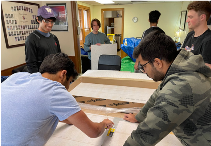
Members of the Spring 2023 Delta pledge class help to cut and install new ceiling tiles in the chapter house living room.
