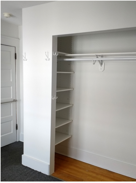
Room 35 renovations, including new closets and storage space designed and built by our contractor.
